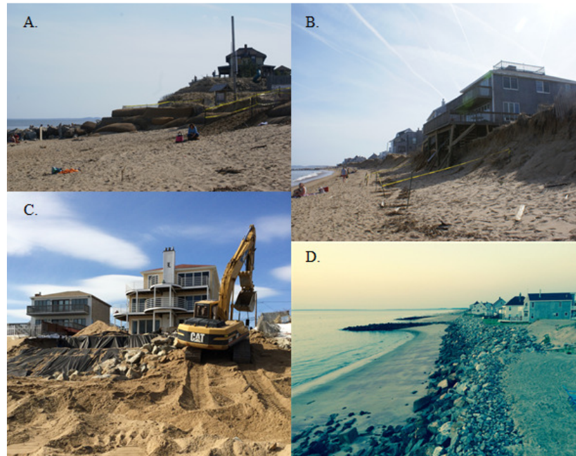
Fig 3 A. Coir bags at Center Island, 2010 B. homeowner stabilizing porch post storm, 2010 C. Revetment construction, two south groins, 2014 D. Groins & rip rap revetment, Annapolis Way, 2014
